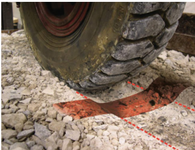
FIGURE 4 Rutting occurs from subgrade soil movement, causing premature deterioration of the roadway or construction platform.
