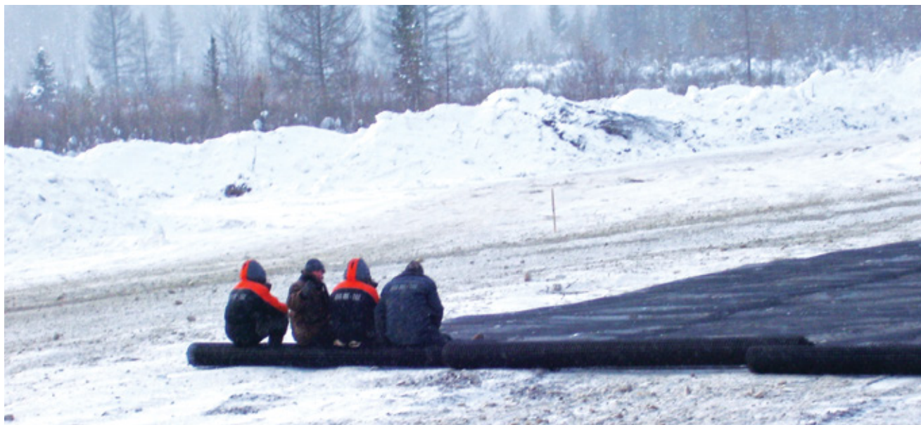
This 2005 project in Siberia demonstrates that geogrids can be installed in near-arctic conditions.
