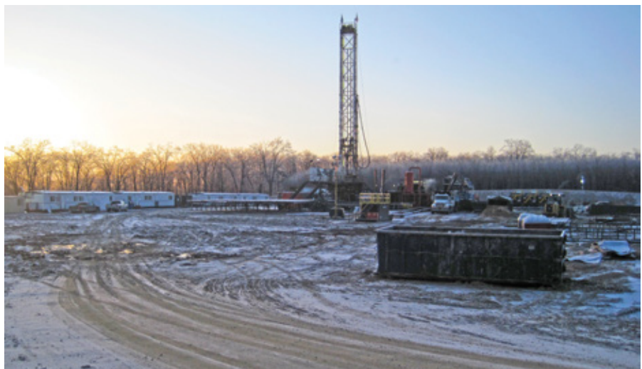
The access road shown in the image above was stabilized with Tensar TriAx Geogrids, while the well pad was not. A dramatic difference in surfaces between the smooth, stable road and muddy, unstable well pad can be seen.
