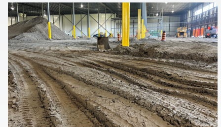
Inside of the warehouse floor experienced major rutting and pumping.
