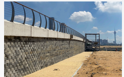
Completed photo of the modular block wall faced reinforced soil retaining wall system in late 2020
